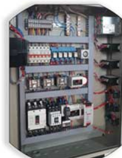
Electrical panel With Complete protective equipment
